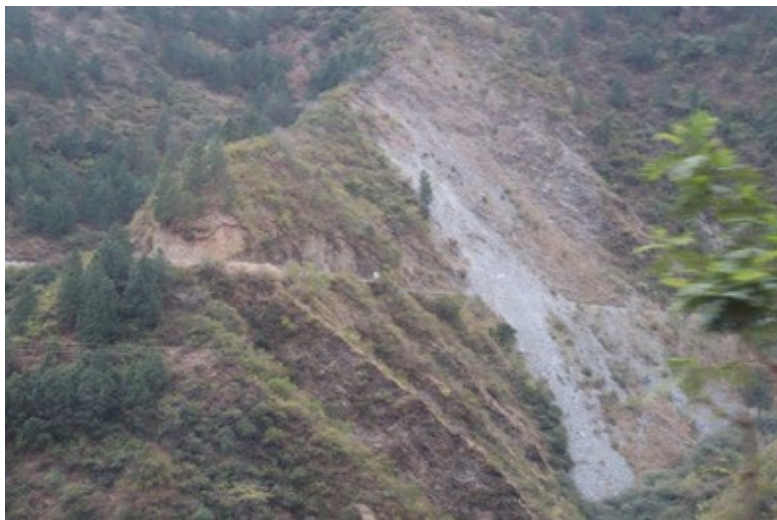
Landslide-prone areas in tourism road
